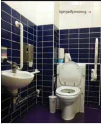
Picture 5.7.1.1 Sample of emergency pull string with two red rings in unisex toilet with left transfer
