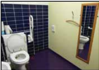
Picture 5.7.11.1. Sample of mirror attached to the wall in front of washbasin in toilet
