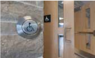
Picture 1.9.5.8.1. Example of electric doors using a switch to open
