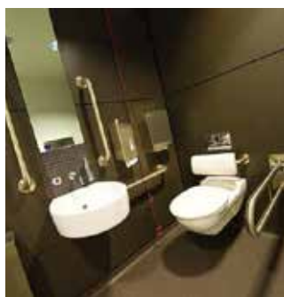
Picture 5.2.1.6. Sample of accessible unisex toilets with transfer on the right-hand side
