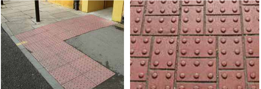
Picture 1.6.1.5. Example of red blister surfaces
