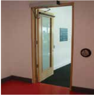
Picture 1.9.5.4.1. Example of the door with fire alarm system
