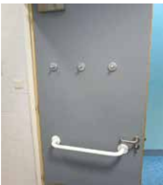
Picture 5.7.5.1. Sample of grab rails attached to the door
