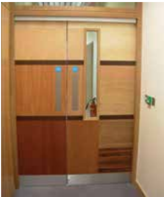
Picture 1.9.5.4. Example of the door which can be opened manually or pushed using the wheelchairs
