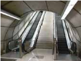
Picture 1.2.9.2. Example of escalators traveling in two opposite directions, a stop button attached to the stair in the center
