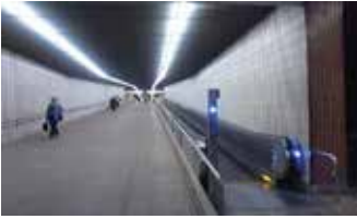
Picture 1.2.10.2. Sample of travelator with signage
