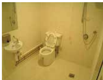
Picture 5.4.2.1. Sample of accessible shower with WC without grab rail and with external pipe.
