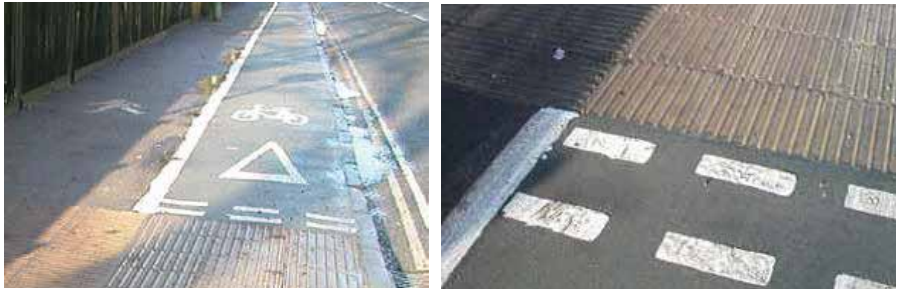
Picture 1.6.2.3. Blister paving surface and corduroy paving surface in parallel with vehicle (bicycle) route (right) and pedestrian pathway (left)
